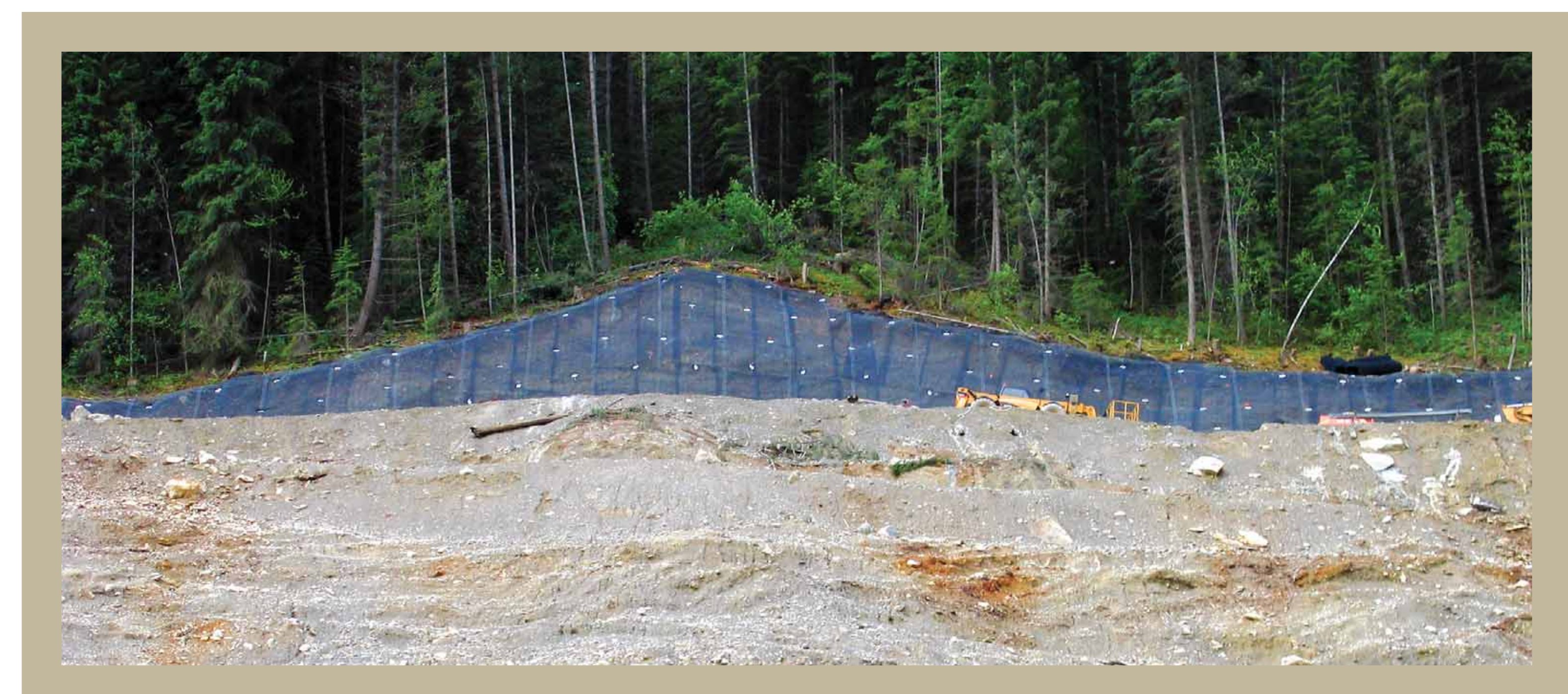
On some steeper slopes, steel mesh is tightly anchored into the soil and underlying rock to prevent surface movement. Seeding follows to provide additional stability.
